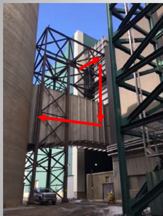
FGD Outlet to Stack
